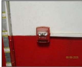
External photo(s) of the production unit(s) Fire alarm bell.JPG
