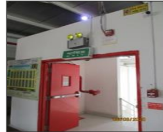
External photo(s) of the production unit(s) Emergency light checked.JPG
