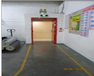
External photo(s) of the production unit(s) Exit sign with light in the fire rated door.JPG
