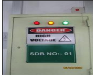
External photo(s) of the production unit(s) Danger sign.JPG
