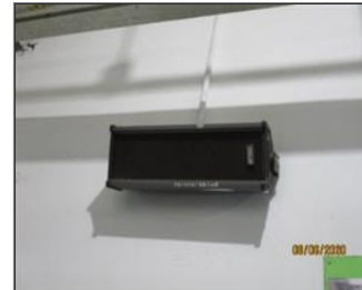
External photo(s) of the production unit(s) PA System.JPG
