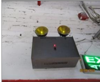
External photo(s) of the production unit(s) Emergency light.JPG
