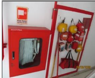
External photo(s) of the production unit(s) Firefighting equipment.JPG
