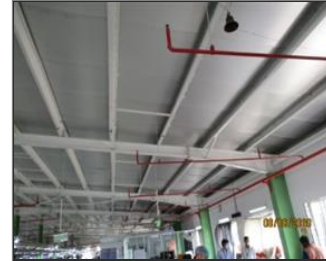
External photo(s) of the production unit(s) Sprinkler system.JPG
