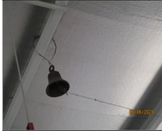
External photo(s) of the production unit(s) Manual fire alarm bell.JPG
